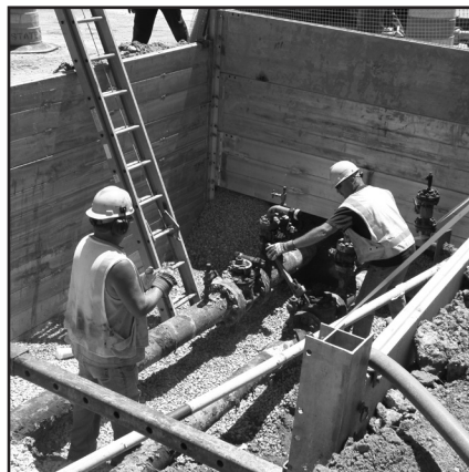
A three-sided configuration with end panels pinned 305 mm up in corner posts allowing gas utility to run through
