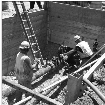
A three-sided configuration with end panels pinned 1 ft. up in corner posts allowing gas utility to run through
